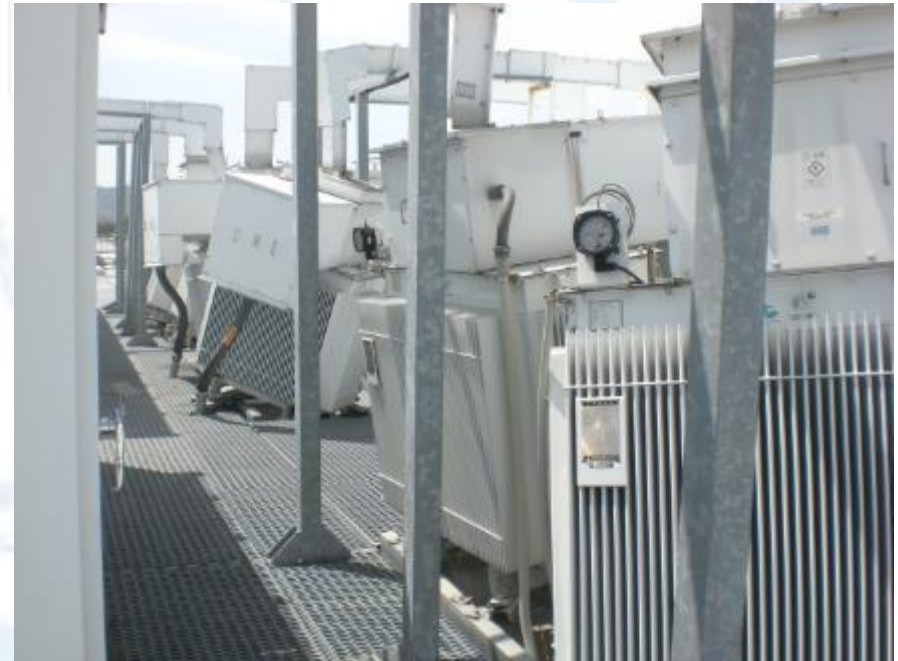
[Transformer tilted by an earthquake]
