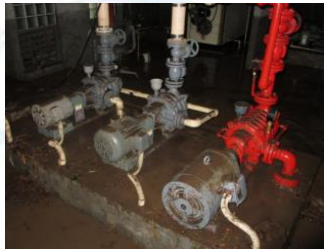
[Motors that have been subjected to flood damage]
