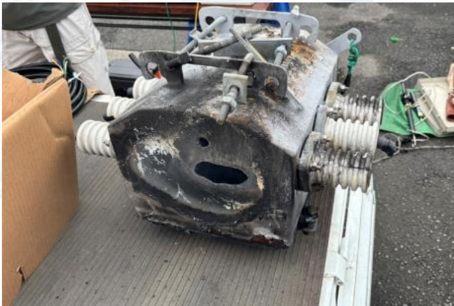
[Switching device burnt by a lightning strike]
