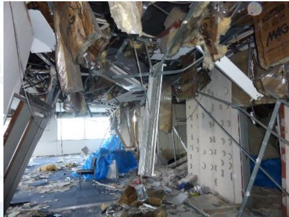
[Ceiling that was dropped by an earthquake]
