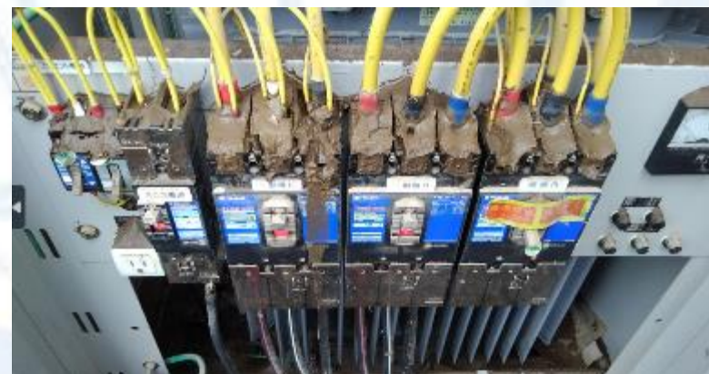
[Circuit breakers that have been subjected to flood damage]
