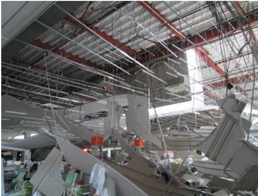
[Ceiling that was dropped by an earthquake]
