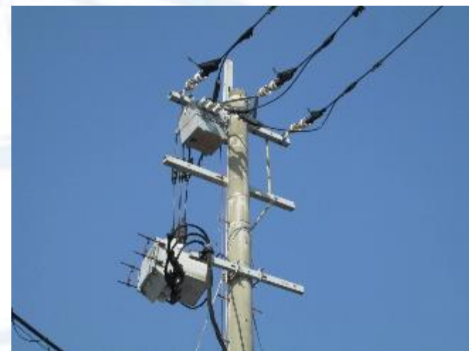
[Instrument transformer removed from its fixation position due to an earthquake]
