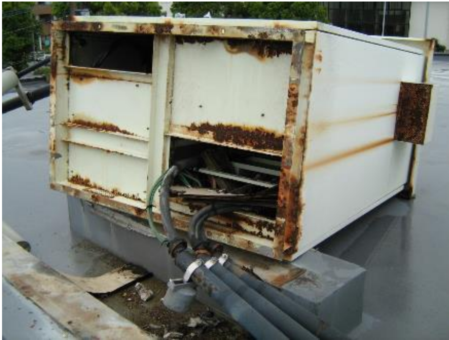
[Cubicle fallen down by an earthquake]
