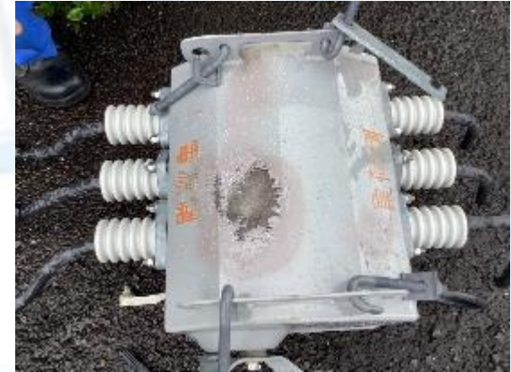
[Switching device burnt by a lightning strike]
