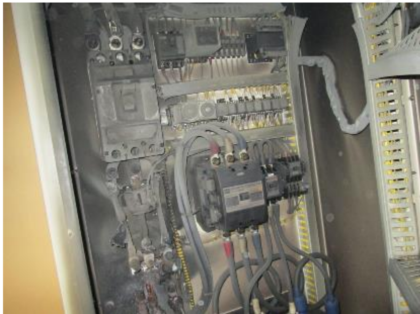
[Distribution panel burnt by the effects of a lightning strike]
