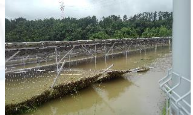
[Flooded solar panels]
