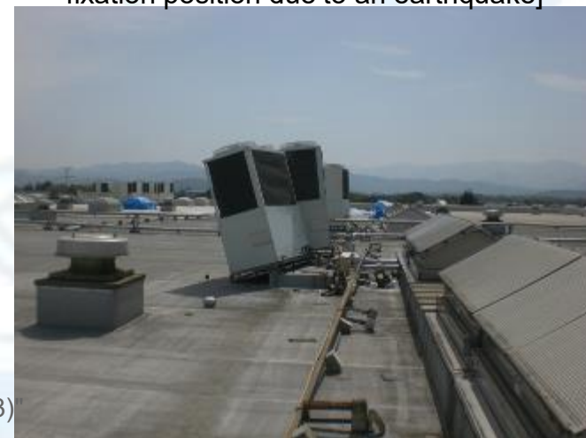
[Air conditioner tilted by an earthquake]
