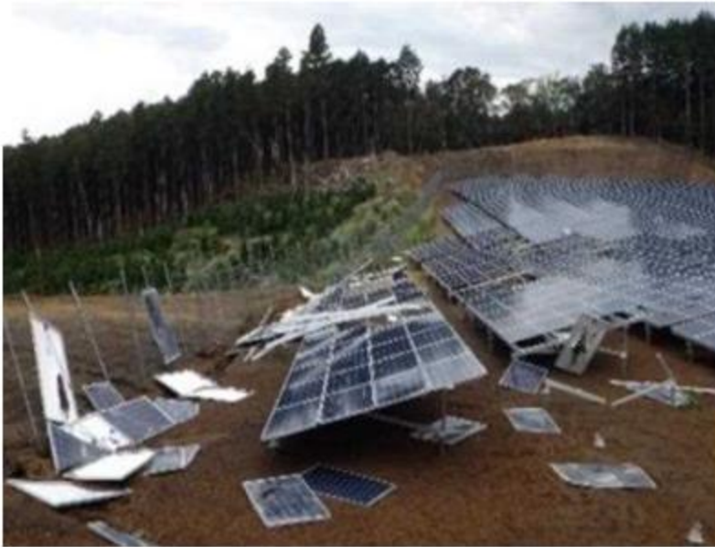
Damage caused by typhoon strong winds
