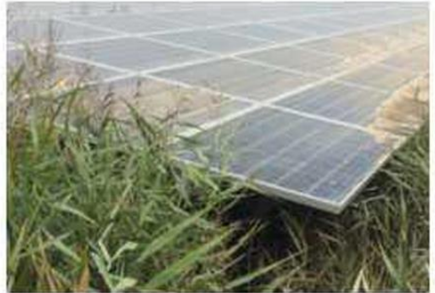
Damage caused by flooding
