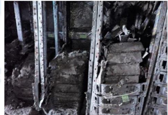
Severely burned batteries Batteries gravement brûlées
