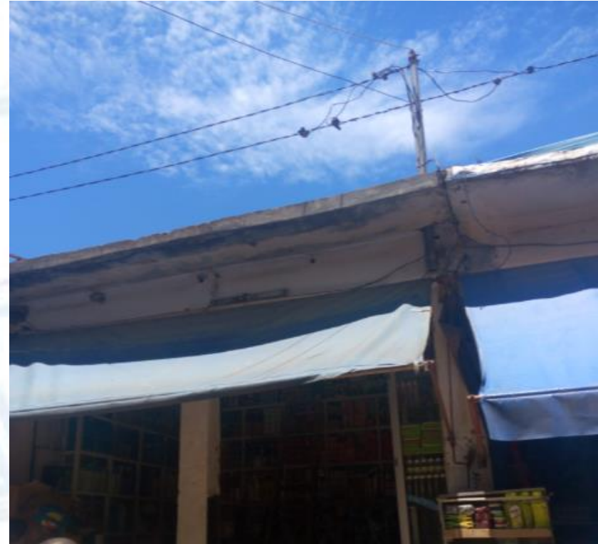
Non compliant installations High risk of non technical losses
