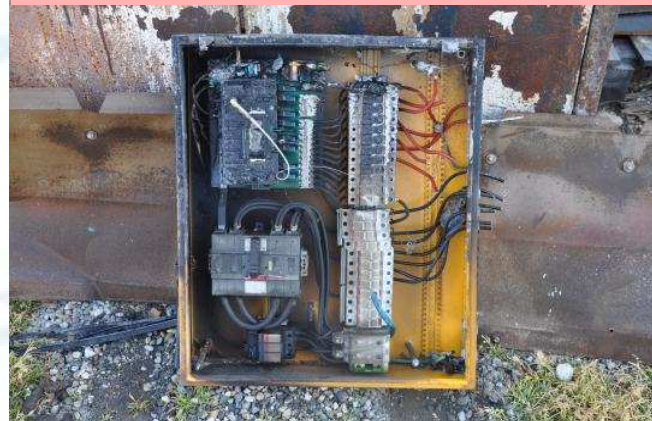
Fires – electrical origin
