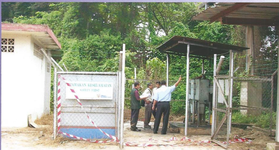
Inspecting exploded ring-main-unit which has caused power cut-off to the nearby residents before being replaced with a new unit.
