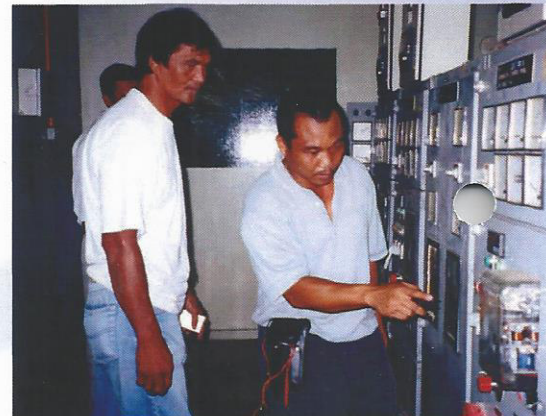
"Competent electrical personnel" is inspecting a protection relay on a Main Switch Board panel.
